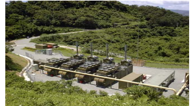
Biogas power plant, Municipal waste landfill, Taipei
