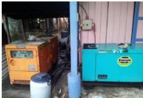
Diesel generators on Pulau Ubin
