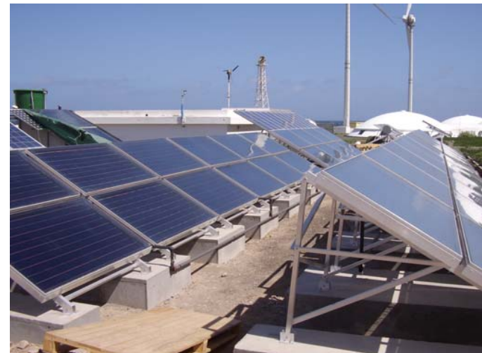
Flat glass solar water heaters
