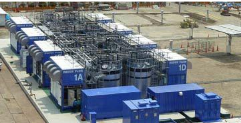
Redox Flow Battery
