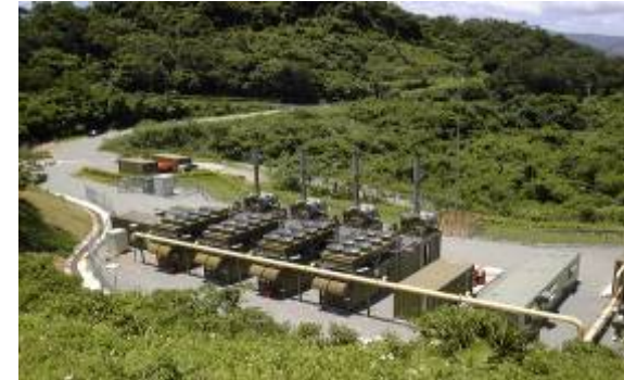
Biogas Power Station Sanzhuku Sanitary Landfill Site Taipei
