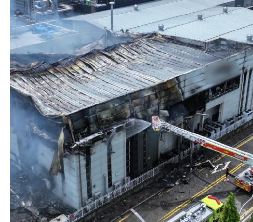
Battery Safety Issues
