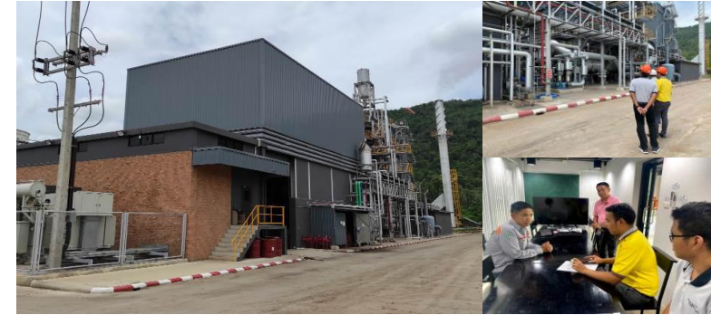
4.9-MW on-grid biomass power plant at Ban Khao Noi, Phitsanulok | commercial power plant
