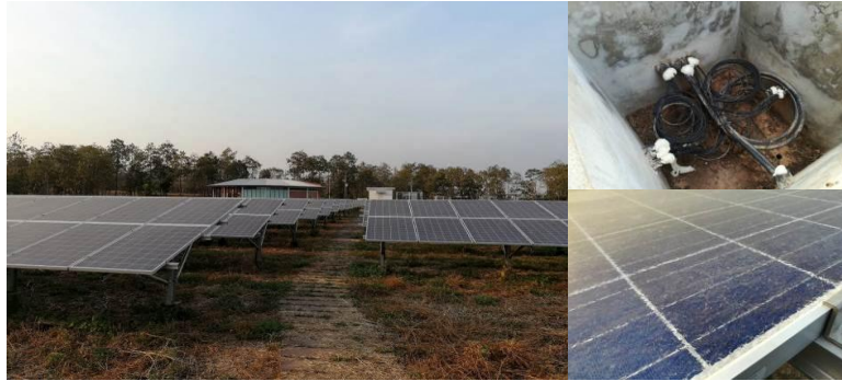
702-kW on-grid solar power plant at CMRU, Chiang Mai | state-owned power plant
