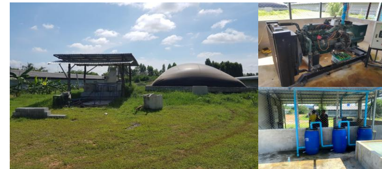
Biogas power plant with 60-kVA generator at Ban Kham Khaen, Khon Kaen | community plant
