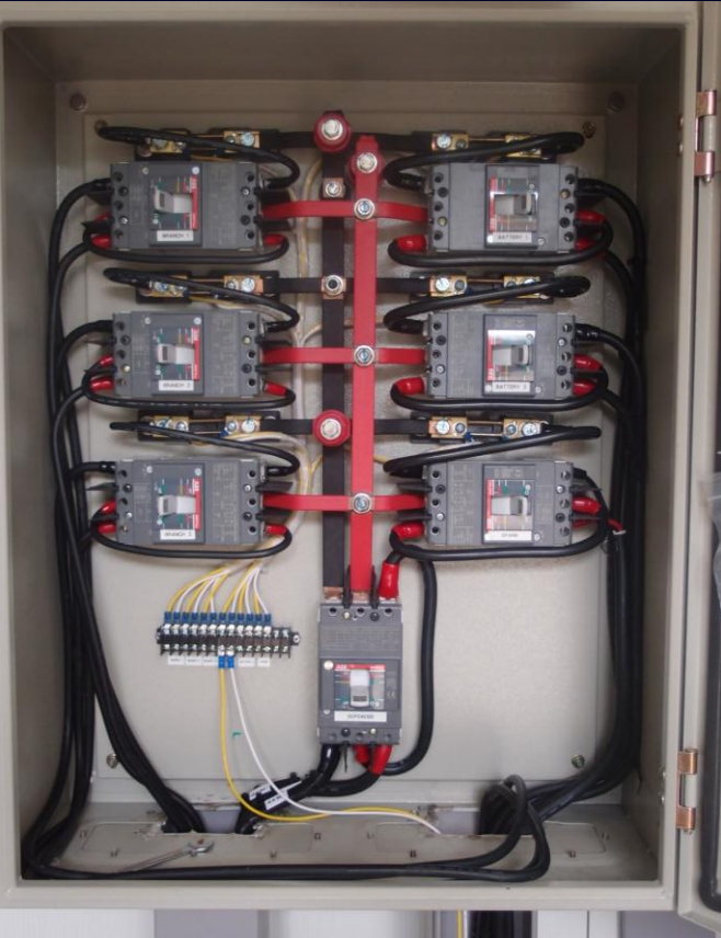
Main Combiner Box
