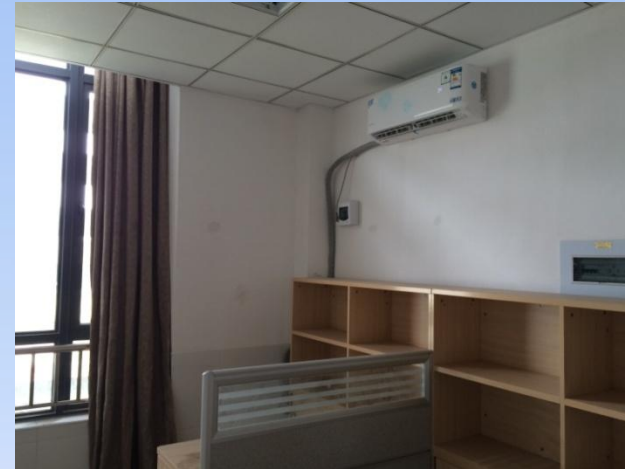
380V DC Air Condition
